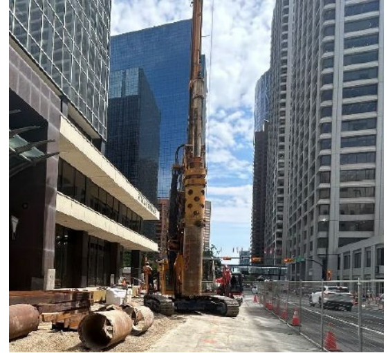
Looking east at Enmax vault installation at 2 Street S.W. and 5 Avenue S.W.
