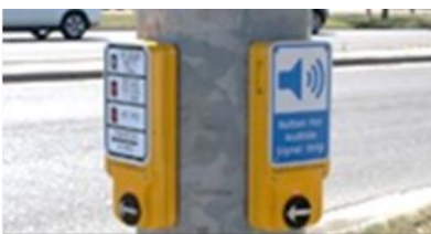
477 Accessible Pedestrian Signals in operation (50 added)
